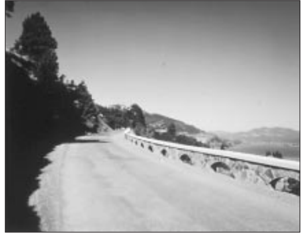
Oregon DOT rehabilitated these stone walls on the Historic Columbia River Highway rather than replace them.
