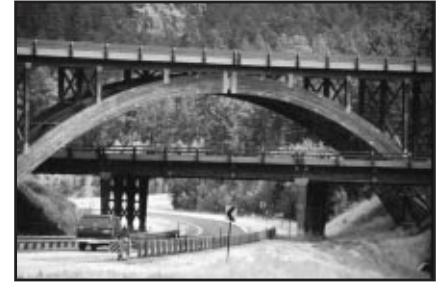
The byway experience starts even before you get on the byway, when you exit the main highway toward Keystone by crossing a laminated wood truss bridge at the 16/16A intersection. It echoes the rough-hewn timbered look that is evident on the byway. The full-color photo is even more impressive - contact Barb Koth if you want that .jpg file.
